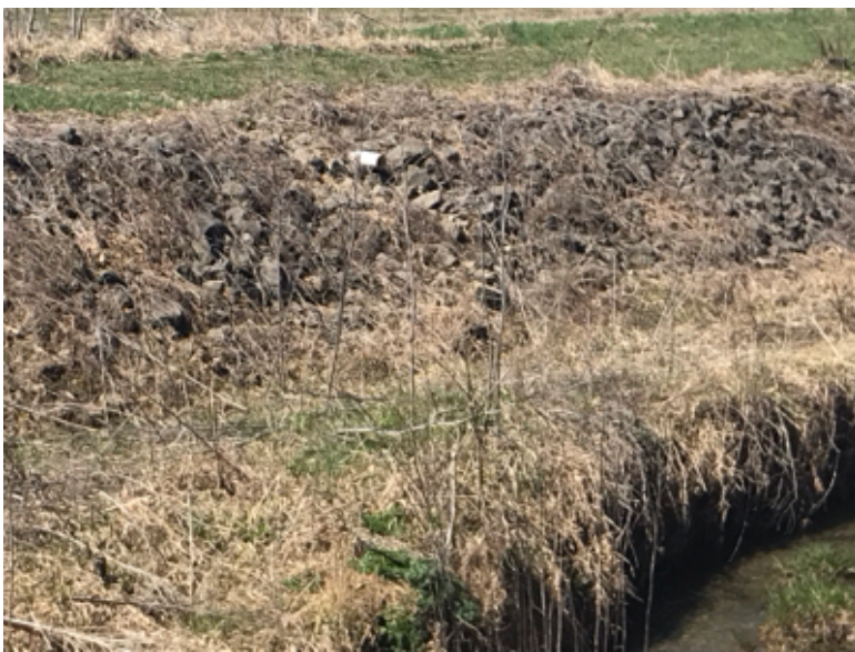
Outfall not mapped
